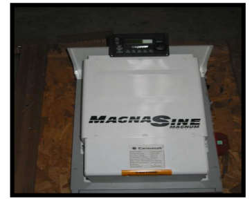
Magna Inverter - E-Panel
