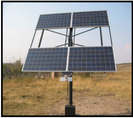
Solar Panels & Tracker
